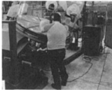
FIG. 7 PLASTIC BAG ENCLOSURE THAT SIMULATES A GLOVE BOX, USED TO PURGE IRREGULARLY SHAPED COMPONENTS IN GTAW OPERATIONS
