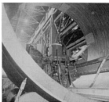
FIG. 38 WELD CLADDING OF A 1.8 M (6 FT) INNER DIAMETER PRESSURE VESSEL SHELL USING 100 MM (4 IN.) WIDE BY 0.64 MM (0.025 IN.) THICK STAINLESS STEEL STRIP. NOTE SMALL "WINDOWS" THAT HAVE BEEN CLAD WITH 50 MM (2 IN.) WIDE BY 0.64 MM (0.025 IN.) THICK INCONEL STRIP. COURTESY OF J.J. BARGER, COMBUSTION ENGINEERING
